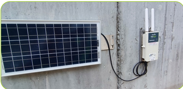
4G Gateway and solar panel installed on bridge wall
