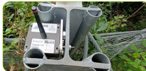
Wireless Tilt Sensors with magnetic mounts installed on steel posts of the rockfall barrier
